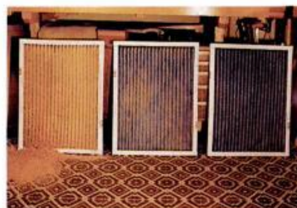
Three-stage filtration. The top filter (left) collects most of the dust, and the other two catch the rest.
