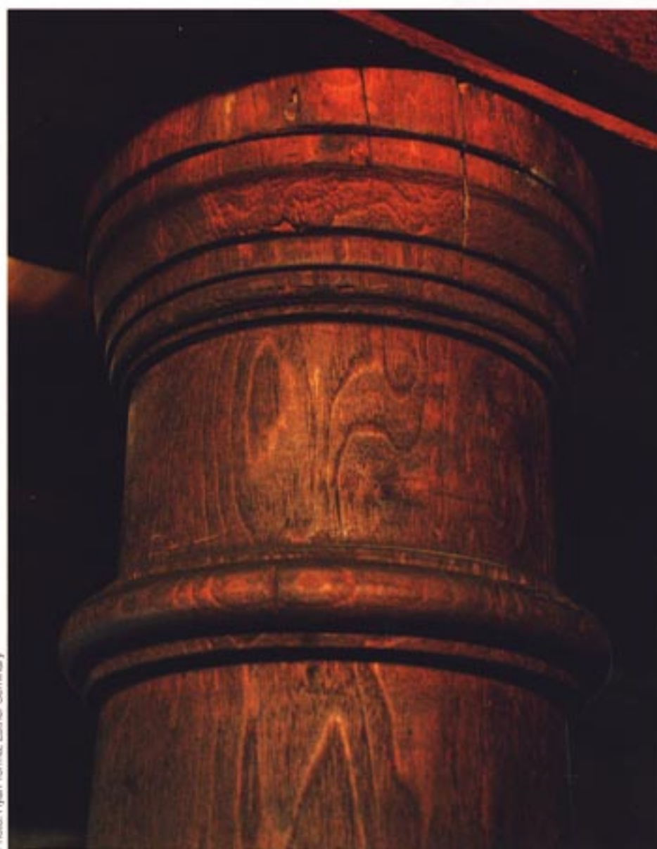
Detail of a column showing tool marks and grain tearout.
