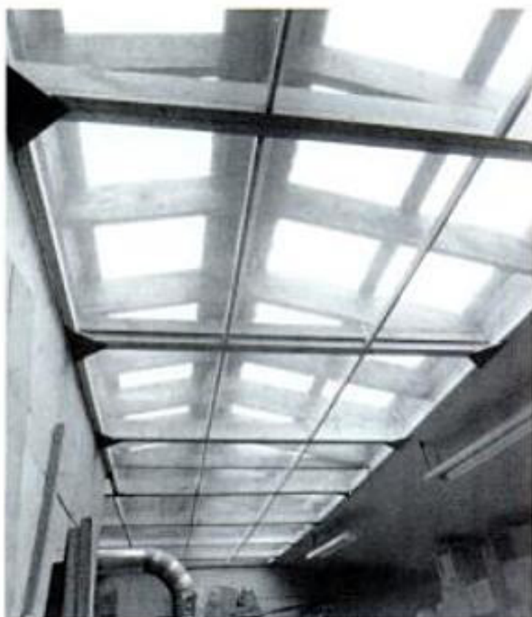
This low-tech, peak skylight runs the length of Michael Elkan's 100-ft.-long Oregon shop and offers plenty of diffuse natural light.
